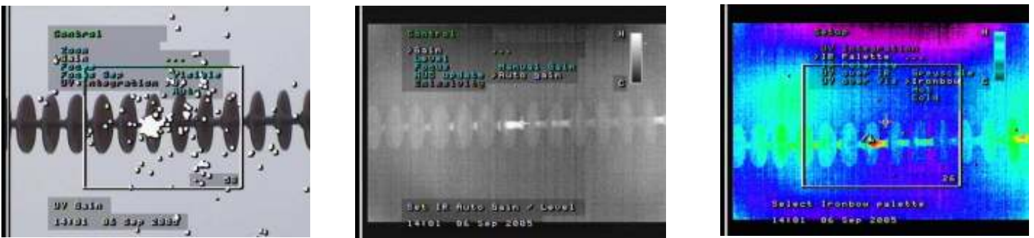
Figure 9: Ultraviolet, Infrared greyscale and UV overlaid on IR images under wet conditions at 120kV, note the increase in corona activities
